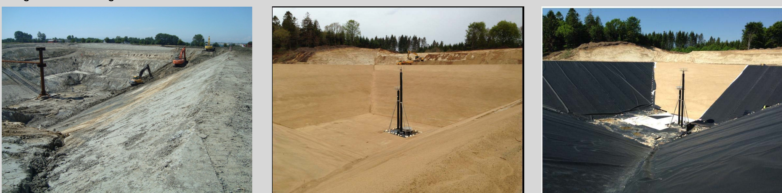
Fig. 7: Pit construction: (a) digging (b) establishing shape (c) lining with plast foil. Source: http://www.solar-district-heating.eu
