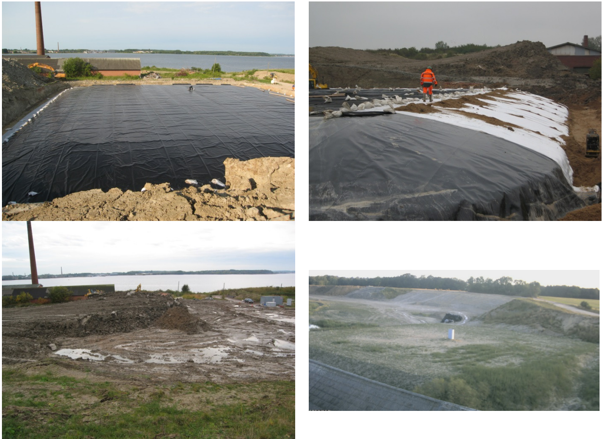
Fig. 3. EM – UPHS test plant at Nybøl Nor, Denmark 2012. Top left: Laying and welding of two layers of 1 mm LDPE membrane. Top right: Laying of geotextile reinforcement. Bottom left: Placing of 3 m soil load (17.000 tons) on the two membranes. Bottom right: Summer 2013, test plant after approx. 100 storage cycles.
