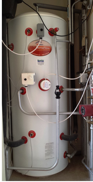
Figure 2.7: Heat storage tank in a smart solar tank system connected to solar thermal collector on building roof.
