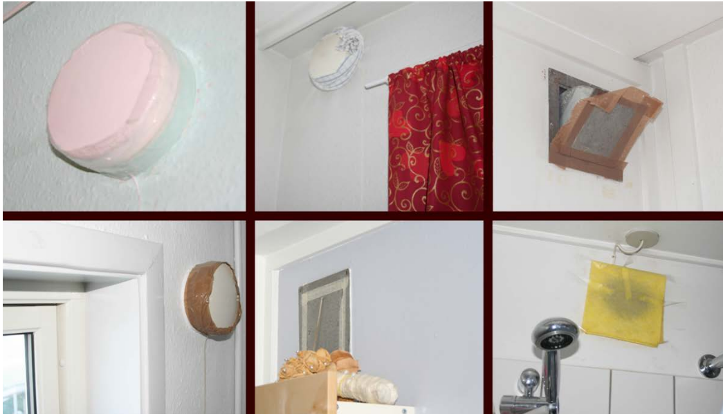
Figure 26. Sealing of the fresh air inlet to avoid cold draft in winter
