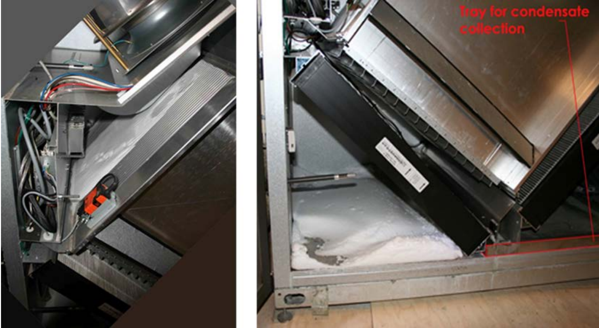
Figure 12. Frost formation in the heat exchanger and snow accumulation in the intake chamber
