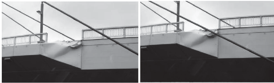
Figure 2.15: Violent cable vibration observed at a certain proto-type cable-stayed bridge in Japan, (Matsumoto et al., 2010).
