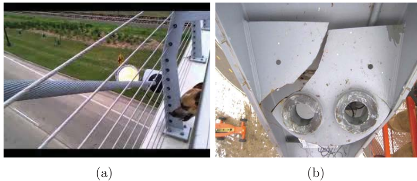
Figure 1.2: Episode of wind-induced bridge cable failure at the Sabo Pedestrian Bridge in Minnesota (Picture from http://failures.wikispaces.com/Cable+Bridge+Failures+Overview ).
