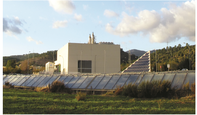
Figure 5. Picture of the Parc Bit plant comprising 900 m 2 collectors, 2 x 1.4 MW e co-generation units and 1.3 and 0.43 MW cool absorption chillers and associated hot and cold stores.
