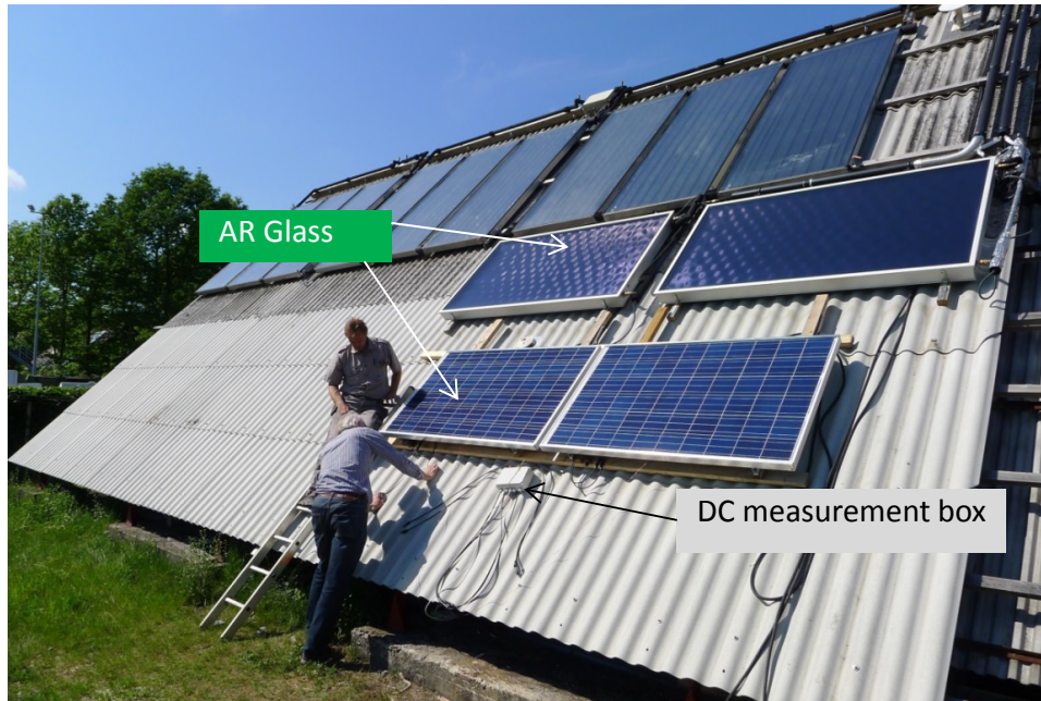
Fig.1. The PV modules during installation in May 2013. Above the PV modules, thermal collectors with the same glass types can be seen.
