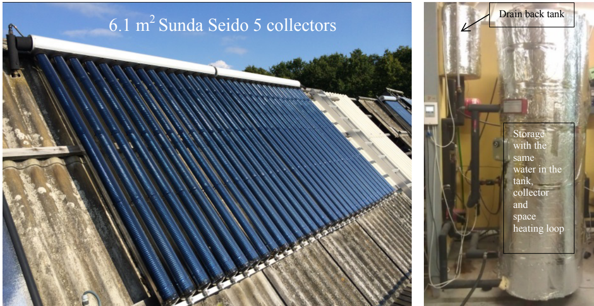
Fig. 3. Lab system at DTU: ETC solar collectors on the roof, storage tank, controller, auxiliary heater and drain back vessel. Note the special single module system to the far right in the first picture. There the same ETC collector was tested with frequent stagnation cycles. This is sometimes told as a problem for drain back systems using ETC collectors. No problems were found after hundreds of cycles.
