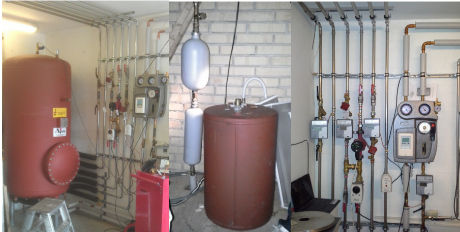
Fig. 6. Top drawing showing the principle for the combination of a drain back and expansion vessel to reduce heat losses. Lower part some more pictures from the demonstration system in Sorø, Denmark. The left picture is before insulation of the storage tank. Note in the middle picture the small drain back vessels (white) and the combined expansion tank (red). Note in the right picture, the pump unit that was convenient to use for the installer, but gave extra pressure drop and malfunction of the combined expansion vessel in the beginning.
