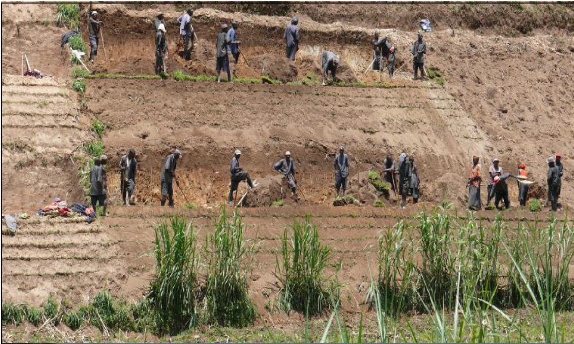
Plate 3. 4: Terracing to stabilize steep slopes at Gatumba (picture taken at Gatumba site)
