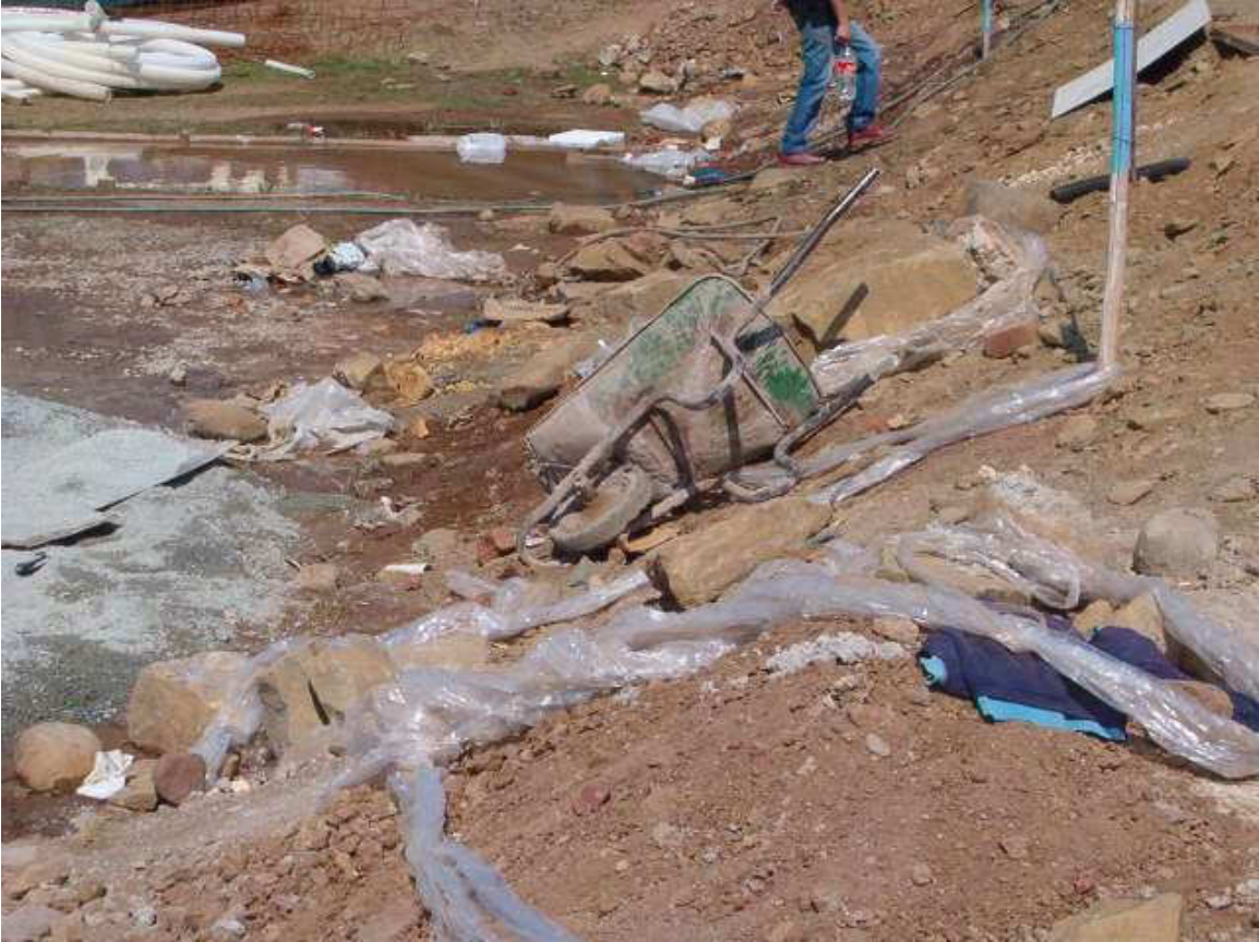
Figure 3-10. Poor waste management during the construction of a fuel station complex in the Lukhanji municipal area.
