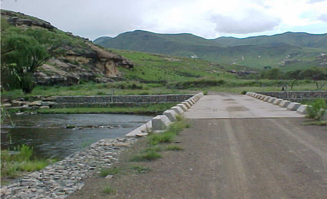
Figure 3-19. Example of a low-impact and low-default project (reconstructed bridge) in the Senqu Municipal area 8 .
