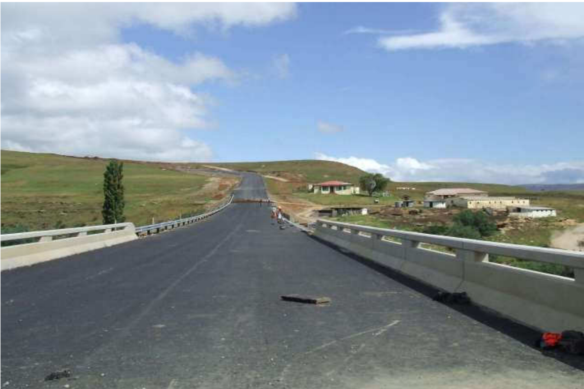
Figure 3-2. The same road and bridge after completion of the bulk earthworks but before all rehabilitation had been carried out.
