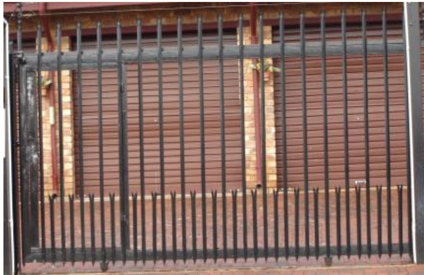
Picture 12: Example of an integrated pedestrian gate
