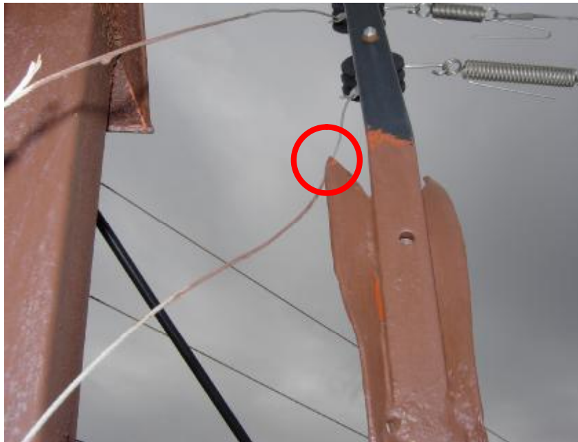
Picture 8: Example of electrified fencing touching palisade fencing resulting in an alarm violation condition
