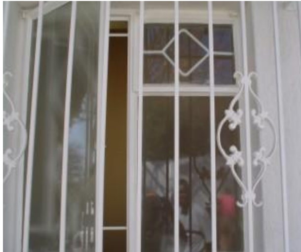
Picture 18: Example of burglar proofing on the outside of the window
