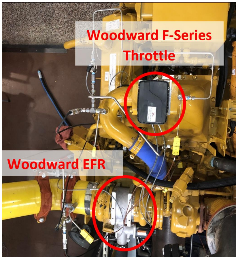
Figure 9: A top-down view of the engine shows the retrofitted Woodward actuators that will give the Woodward Large Engine Control Module (LECM) customizable control of engine operation.
