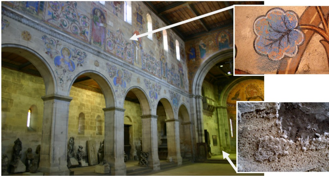
Figure 5-3. Detailed view of damage: paint deterioration in upper level and salt damage in lower walls (Krüger et al. 2010)
