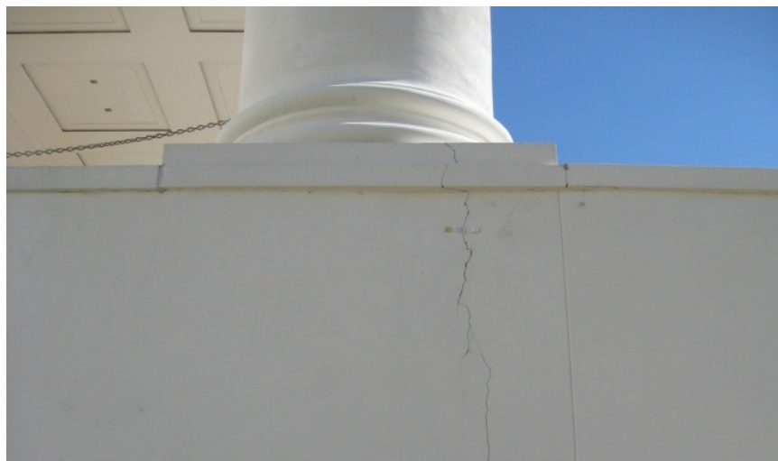
Figure 1-2. Cracking of foundation under column at Virginia State Capitol (Staley 2008)
