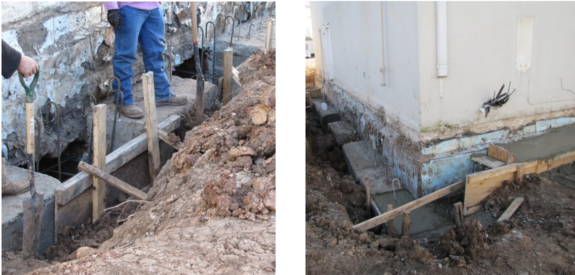
Figure 4-5. Foundation excavations and new footing (left, St. Paul Lutheran 2010) and footing with beam stiffener (right, St. Paul Lutheran 2010)
