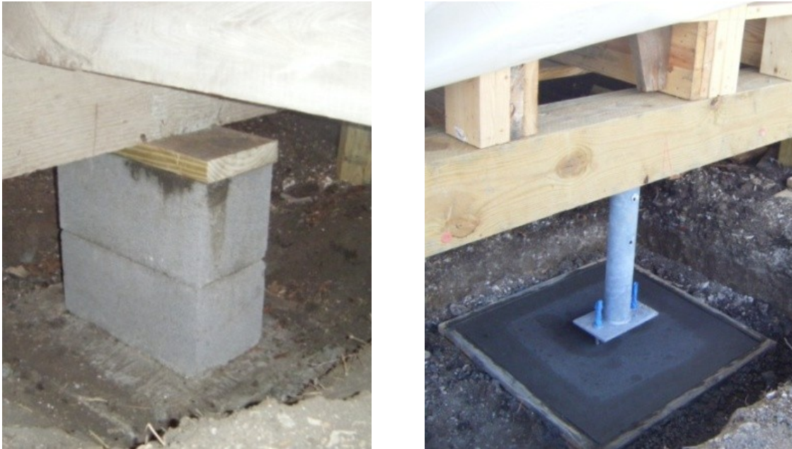
Figure 3-4. Interior span CMU foundation on concrete pad (left) and exterior span steel pedestal on concrete pad (right)
