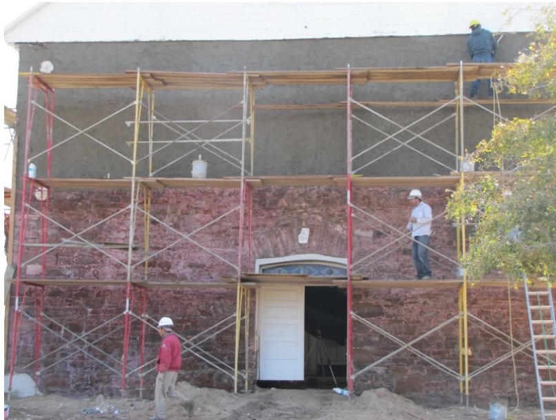
Figure 4-7. Front entrance partially replastered (St. Paul Lutheran 2010)
