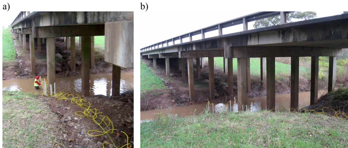
Figure 3.6 (a) View of profile BG14 at bridge 14 carried out in water-covered environment. (b) A profile placed coincidentally with and row of concrete pile foundations.
