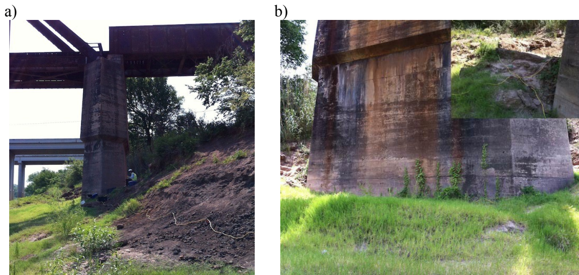
Figure 3.20 View of data acquisition at railway bridge over Brazos River; (a) profile RWB1 electrode were aligned parallel the river and (b) view of foundation and the intersected point of two profiles near the foundation (inset).
