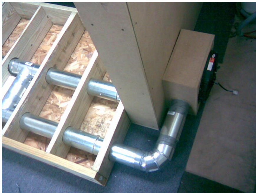
Figure A.4. Connection of the fan to the Comfort Station for the test run.
