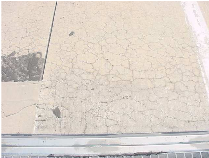
Figure 9 Map-Cracking and Misaligned Trench Drain at Holloman AFB
