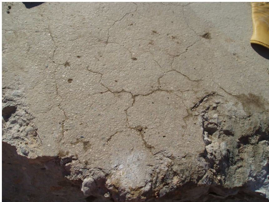
Figure 2 Map-Cracking of Pavement Surface for Edwards AFB
