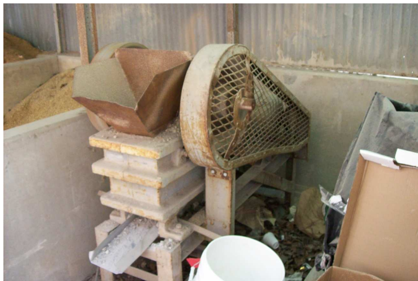
Figure 5 Jaw Crusher Used to Crush RCAs
