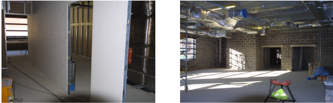
Fig. 3: Plasterboard stud partitions (left) and block wall partitions (right) used in the prototype composite floor from phase 2
