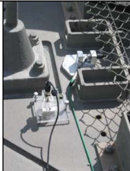
Figure 4 Hanger termination and biaxial accelerometers
