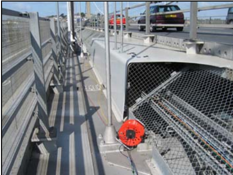
Figure 3 Hanger connection, shear box and cabling
