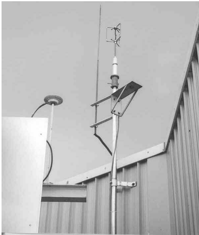
Figure 9 GPS rover antenna and sonic antenna on corner of roof parapet, location 3 of Fig. 1
