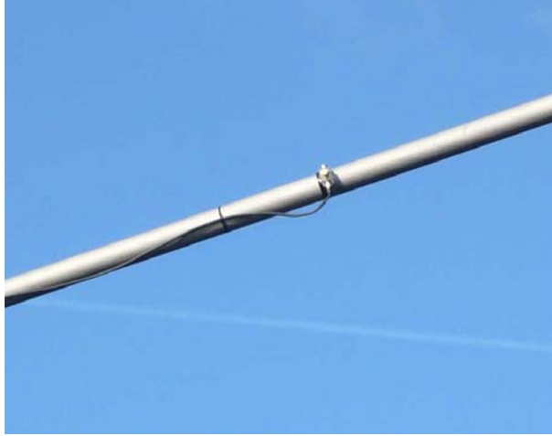
Figure 14: Biaxial accelerometer on stay cable.
