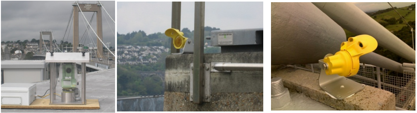
Figure 5: RTS unit on control room roof (left) and reflectors on Plymouth side tower (middle) and Saltash Tower (right).
