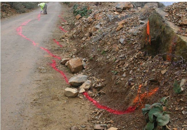
Figure 5. Cracks in the western quarry access road being marked out in January 2011 to aid the identification of further movements.
