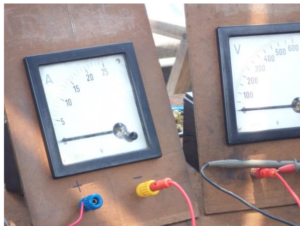
Figure 139 - The Amp and Volt meters.
