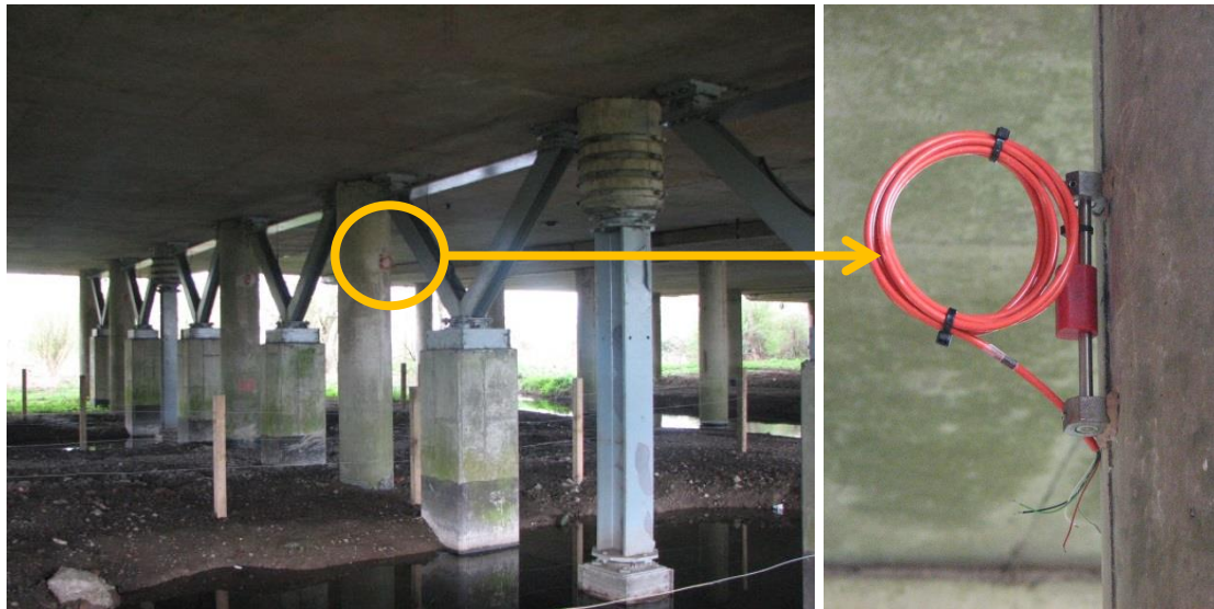
Figure 6.75 Sensors installed on the vertical grid-line S (left) and vibrating wire strain gauge (right).
