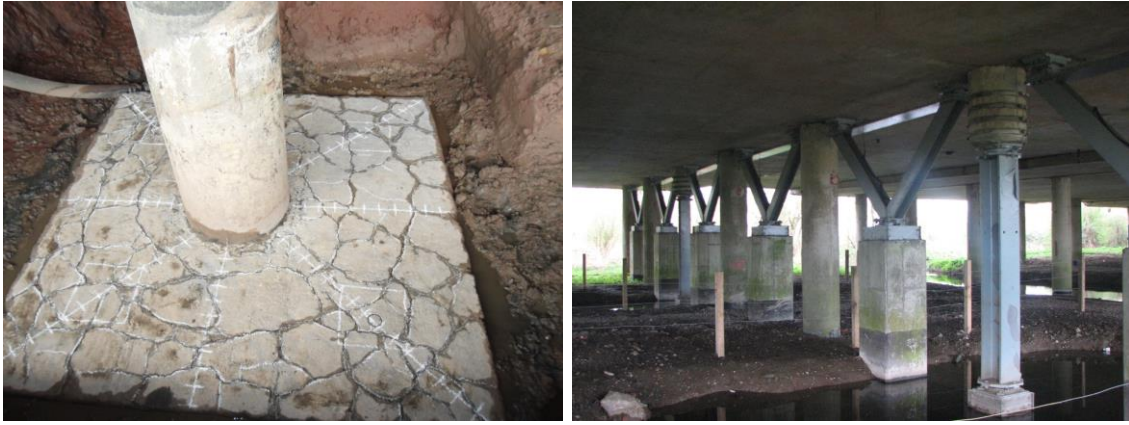
Figure 6.62 Alkali-silica reaction on a footing of a pier of Floodplain #2 (left) and piers subjected to full scale tests on the grid-line S (right). (Courtesy Highways Agency.)
