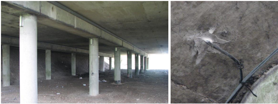
Figure 6.63 Vibrating wire strain sensors (left) and a thermocouple (TH-2) installed on the River Trent Bridge.
