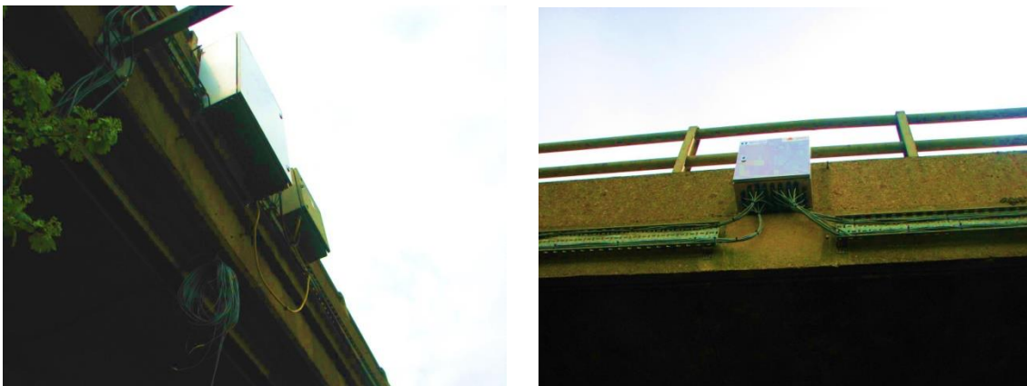
Figure 2.2 Data acquisition and transmission stations on the River Trent Floodplain Bridge. Courtesy Highway Agency.
