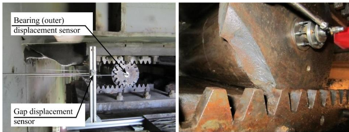
Figure 6.82 Instrumentation for measuring east bearing and east gap displacements (left) and sensor connection to a bearing (right). (Courtesy: Bill Harvey Associates and Pembrokeshire County Council)
