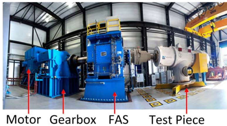
Fig. 2. Typical test setup for Nautilus test rig
