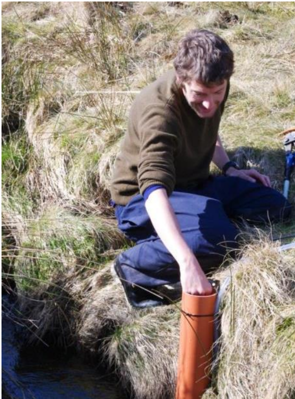
Figure 3.12: Author installing stage monitoring in the main channel at Aclands prior to flume installation.
