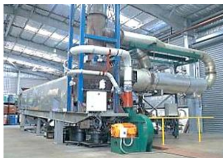
Figure 3.1.1 EESTech Inc. rotary kiln VAM/coal system, (by permission of EESTech Inc.)
