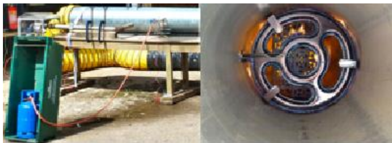
Figure 13 Burner gas supply left and ignited burner right.
