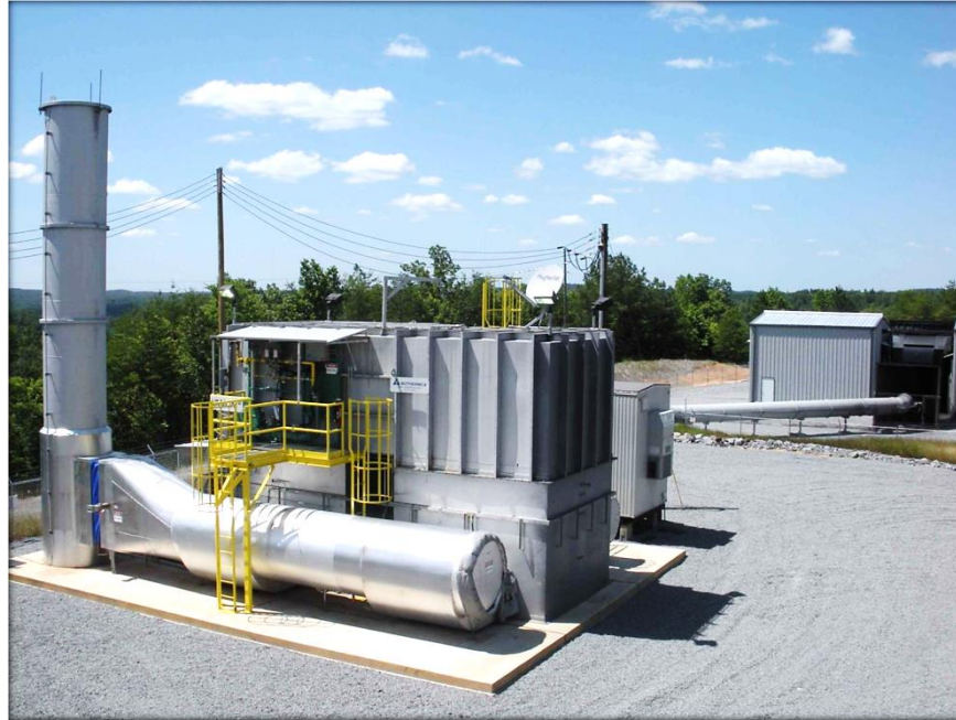
Figure 3.2.5 Biothermica VAMOX® technology (Courtesy, Biothermica 2013)
