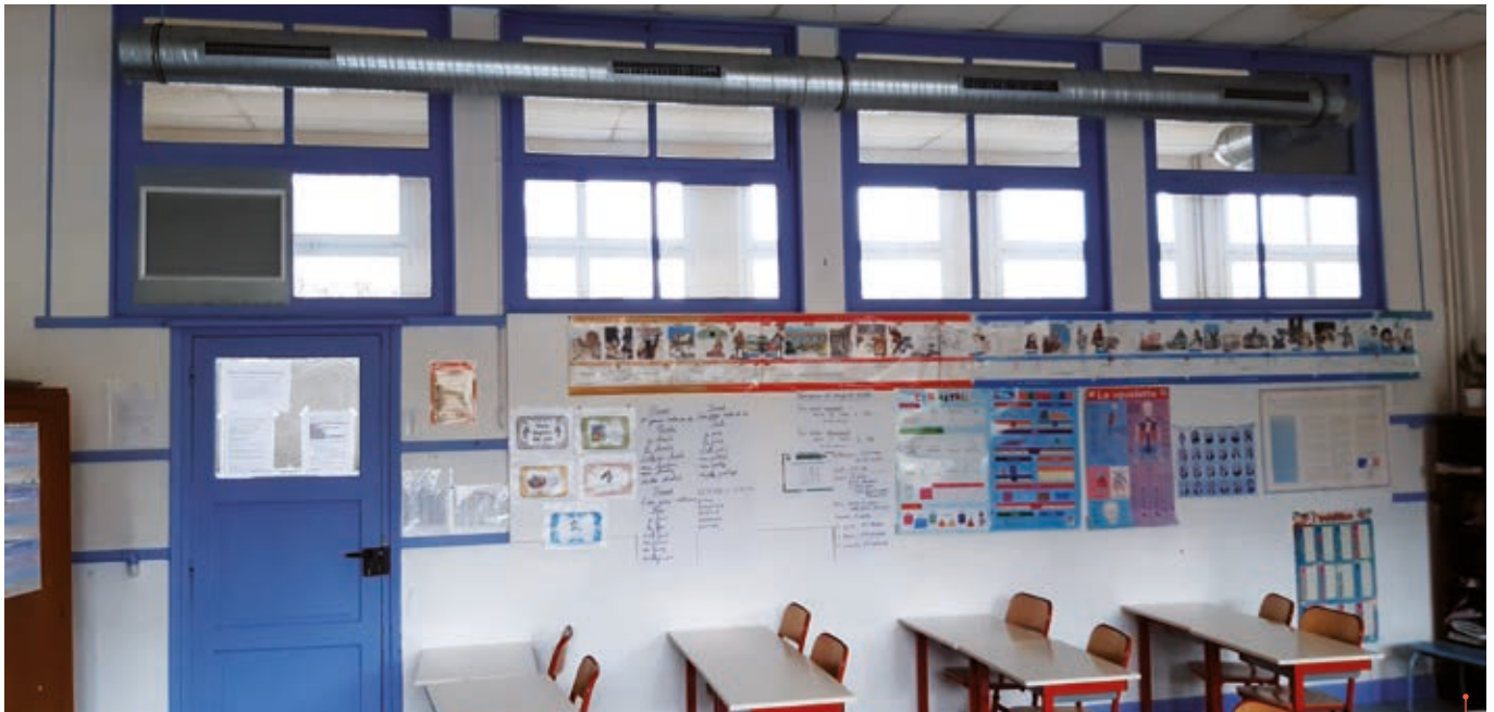
Semi-centralised dual-flow air handling unit, La Fontaine elementary school (Le Raincy, France), class number 3 - © Jade Lachery
