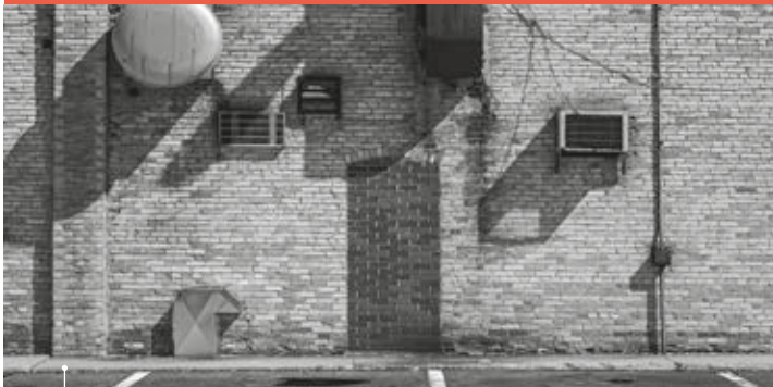
Ventilation units on a building façade
