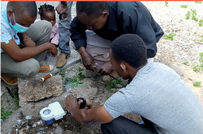
Demonstration of smart meter installation - ©UNTAPPED
