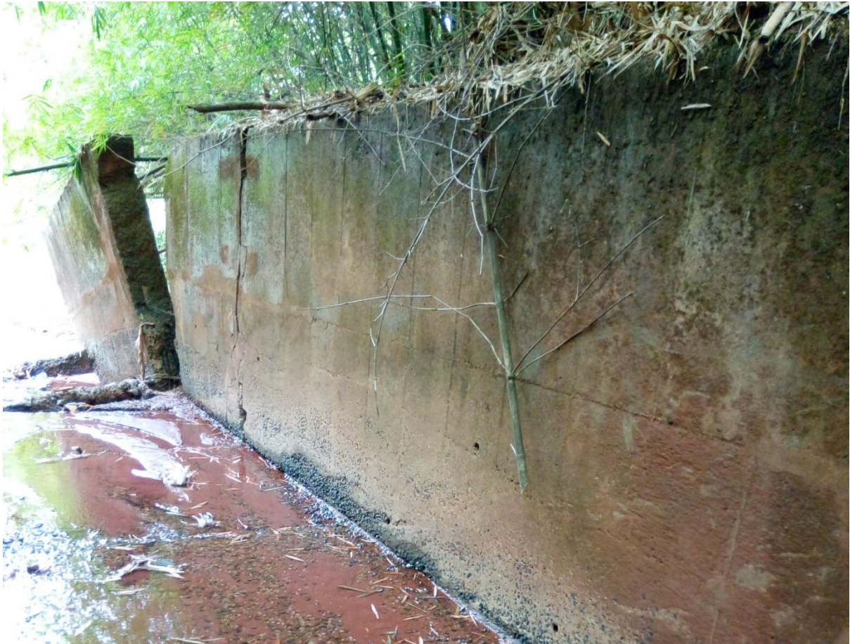
Figure 7.3: Drainage channel constructed by the Federal Government in Amucha in 1983/84 as a gully-control. Some parts of the structure are under threat of collapse as shown in this image and this condition has residents of the community worried.
