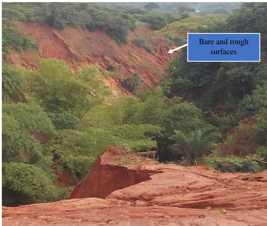
Figure 6.9: Gully site showing presence of bare and rough surfaces which can serve as surface runoff channels. Location: Umueshi, Ideato South LGA, Imo State (photo captured in April 2016).
