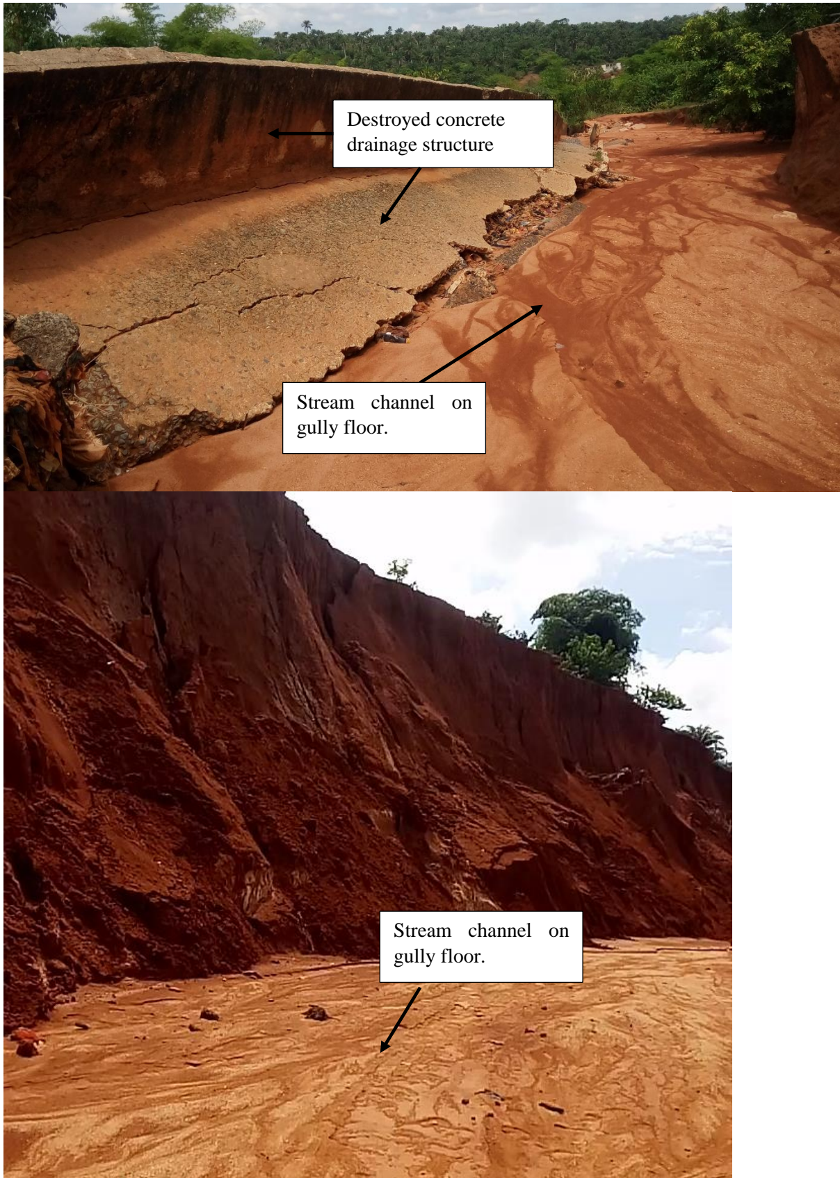
Figure 6.13: Evidence of streamflow on gully floors at the younger Obibi-Ochasi gully. Also shown is a destroyed drainage structure designed to transport runoff to a local base level.
