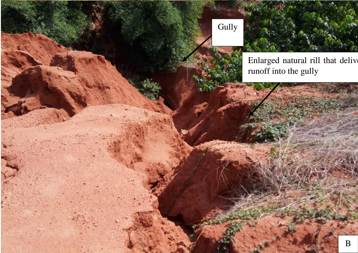
Figure 6.12: Human-made structure and natural rills deliver surface runoff directly into gullies. A) Obibi-Ochasi Gully2. B) Umueshi Gully. Concentrated runoff flowing on gully floors can remove toe support at landslide sites, hence, enhancing slope failure. Natural rills found close to gullies had depth ranges between 0.4 – 0.7 m, widths varied between 0.25 & 2.2 m while lengths ranged from 10 – 60 m.
