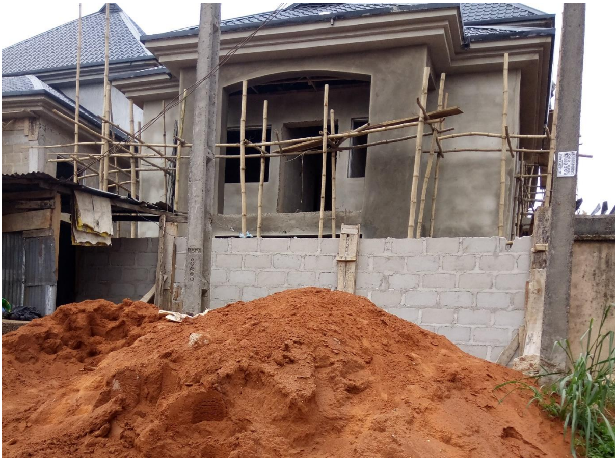
Figure 7.4: Bamboo sticks used for building construction. One of the numerous uses of the bamboo which is a cash-crop.
