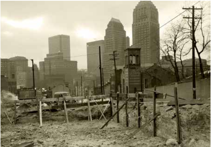
Buildings being torn down in the Lower Hill District as part of Pittsburgh's renaissance and urban renewal programs. The city skyline is visible in the background. January 2, 1957.
