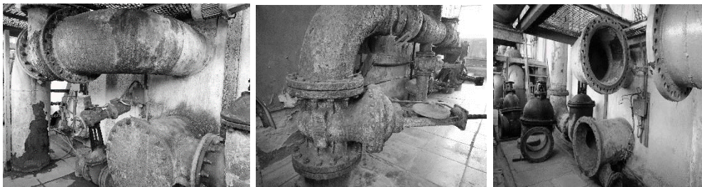
Fig. 4. General appearance of pipelines and valves.
