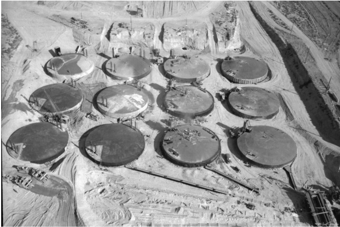
Figure 3. Hanford's underground stage tanks. Source: United States Department of Energy, 2013.
