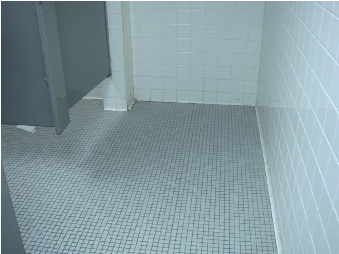
AISJ School - Toilets
