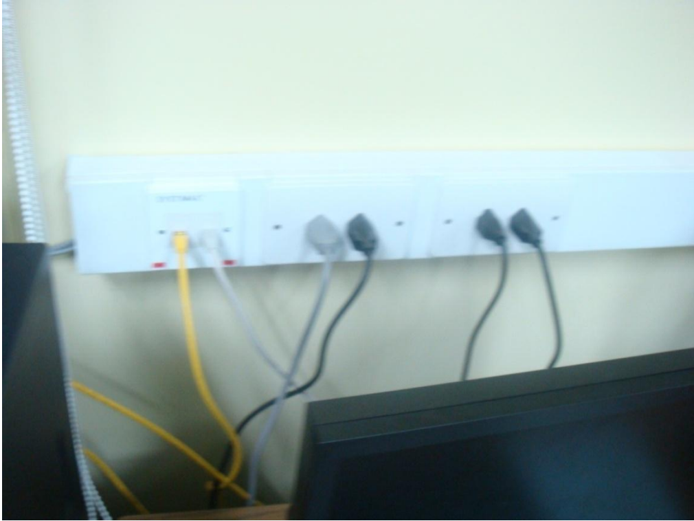
Exposed wiring and easy access for students – Safety hazard
