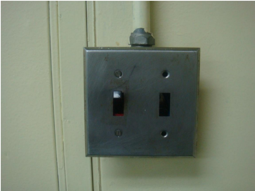
Out dated electrical systems. Damaged electric socket.
