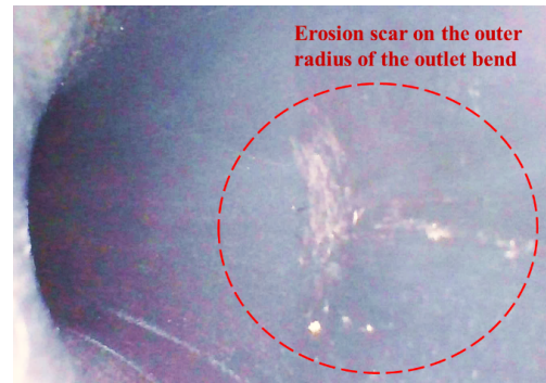
Fig. 13. Photo of observed erosion scar from the tube.
