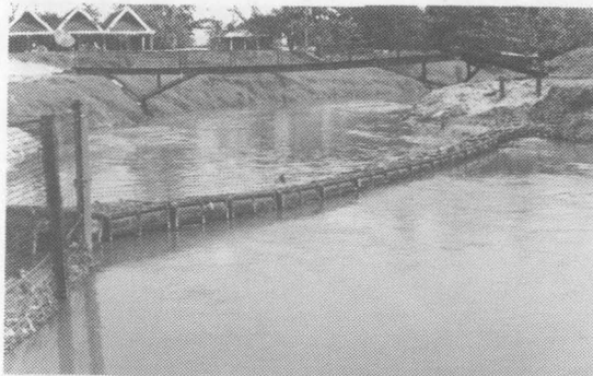
Plate 1: The floating lock boom installed across the Gombak River to trap floating garbage.
