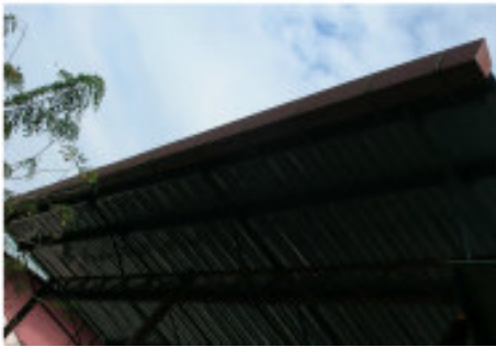
Figure 4: Picture of 140 mm x 140 mm gutter.
