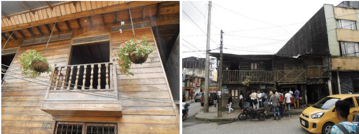
Figure 2. Fieldwork on timber houses in Quibdó: key characteristics in the very well preserved Casa Copete (Carrera 5 & Calle 27) and the UTCh students during condition survey at neighbouring Casa García.
