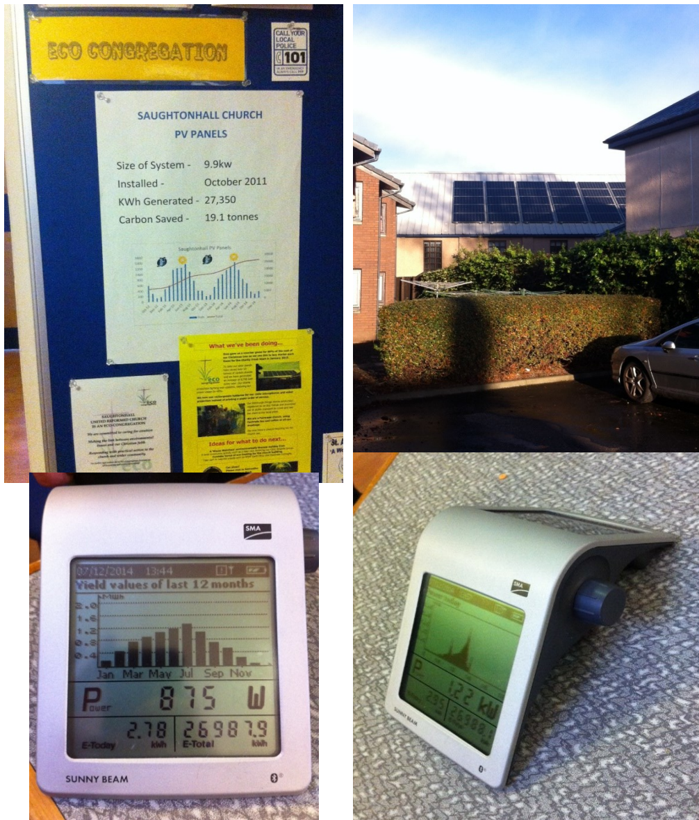
Figure 5.3. Clockwise from top left: the ECS noticeboard displaying ongoing electricity production; a side-view of solar panels on the church roof; the controller indicating hourly electricity production (over a 24 hour period); controller indicating monthly electricity production. The controller also shows the amount of revenue per day/per year, and the total amount of electricity produced since installation.
