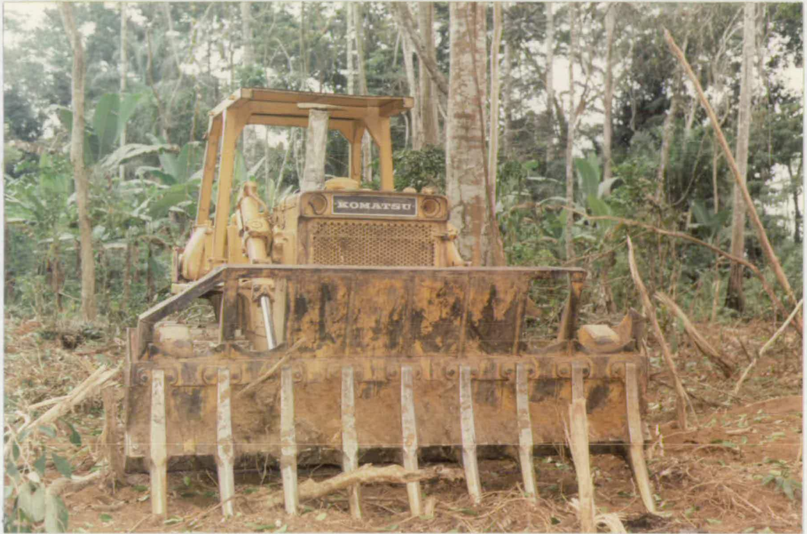
Plate 2: The 23.51 tonnes, D8 straight rake, bulldozer used in the clearance of the Mechanical Regrowth and Complete Clearance plots. Topsoil displacement was mostly by the felled slash and trees being pushed to form windrows.
