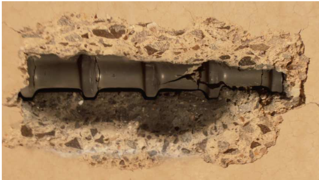
Figure 5.38: Exposed section of grouted duct after Test B.1 on exposed soffit.
