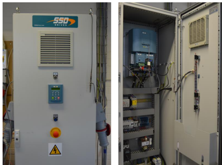
Figure 6.22: Variable speed AC drive – Parker SSD Drive
