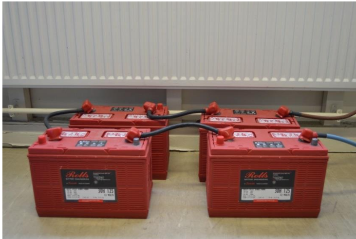
Figure 6.4: Rolls lead acid batteries
