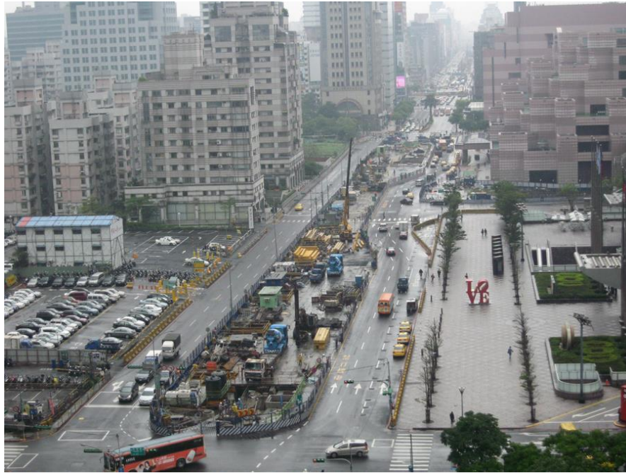
Figure 8.17: A whole view of World Trade Centre Station which is under construction since 2002-2012 (by MRT construction team).
