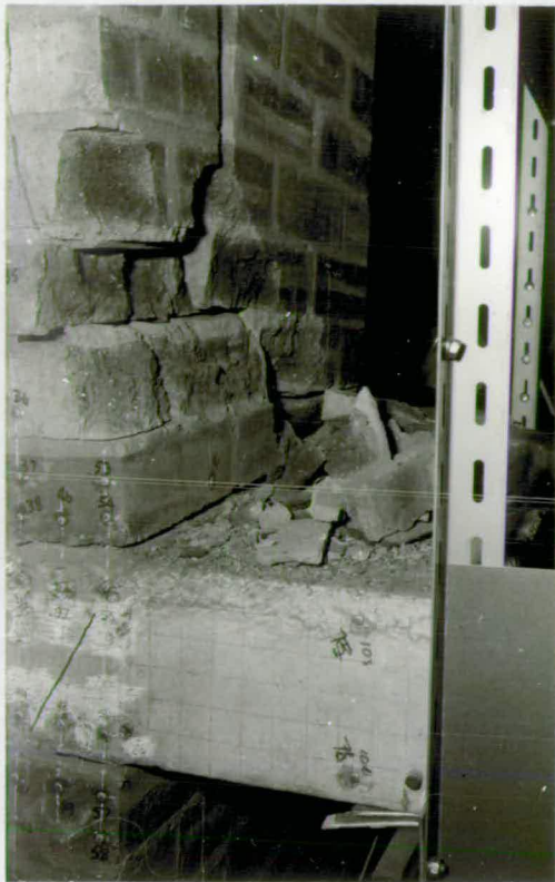
Figure 6.6 Wall and Slab Failure. 1:1/4:3 Mortar Wall Precompression 600 lbf/in 2
