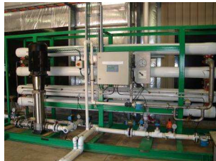
Figure 3 Backup RO unit constructed in 2001
