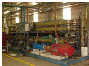
Figure 2 RO unit constructed in 1985
