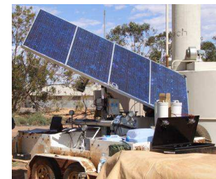
Figure 7 PV powered hybrid UF/RO unit used in this trial.
