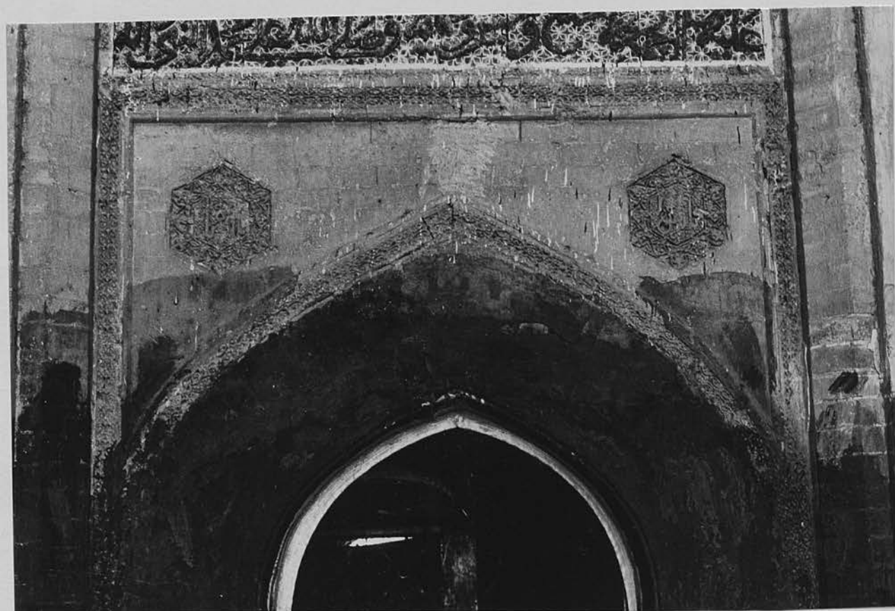
53a. Al-Jadīda (30 km. N.E. of Baghdad): mausoleum of Muhammad al-Sakrān. Brick ornament above the doorway.
