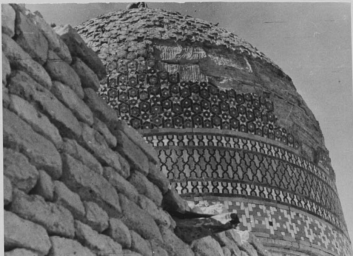
157a. Basra. Jāmi' al-Kawwāz: exterior of dome showing detail of the tile decoration.
