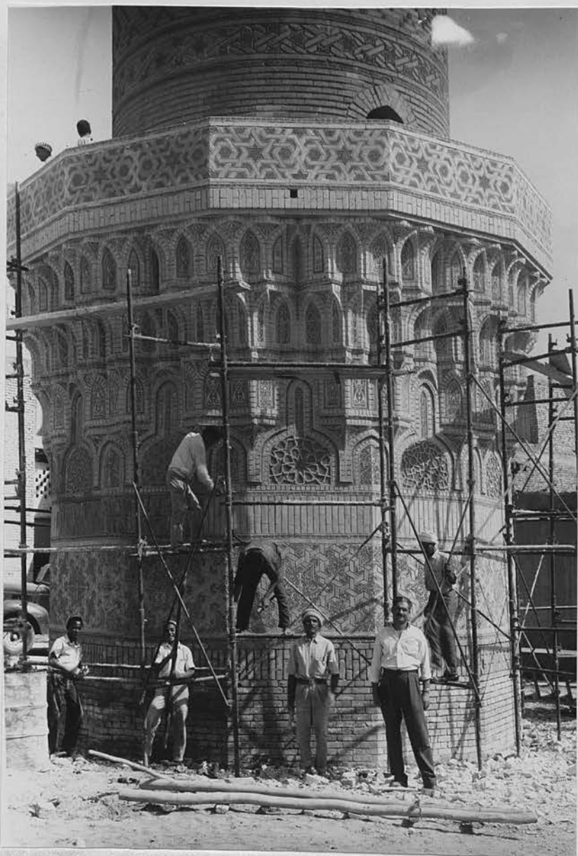
63. Baghdad. The minaret of Sūq al-Ghazl: brickwork of the base, after restoration.
