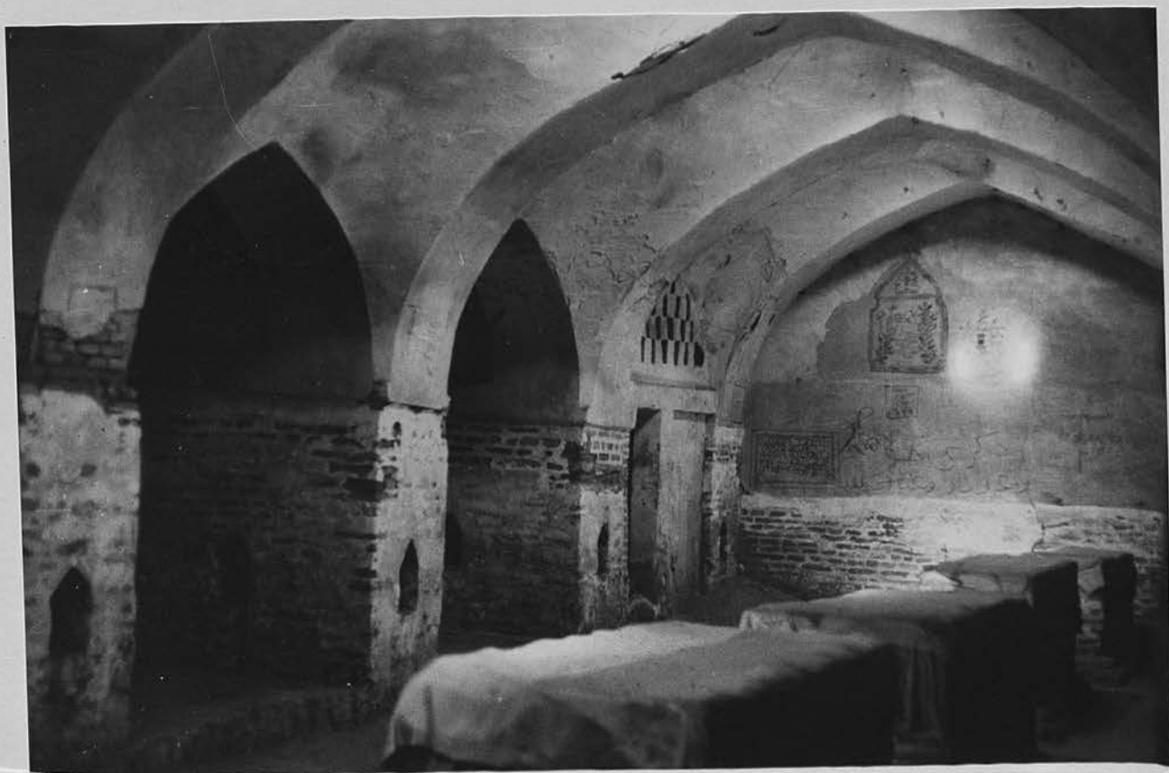
79b. Al-Kifl. Hall behind the mausoleum of Dhū 'l-Kifl: interior, detail of vaulting system.
