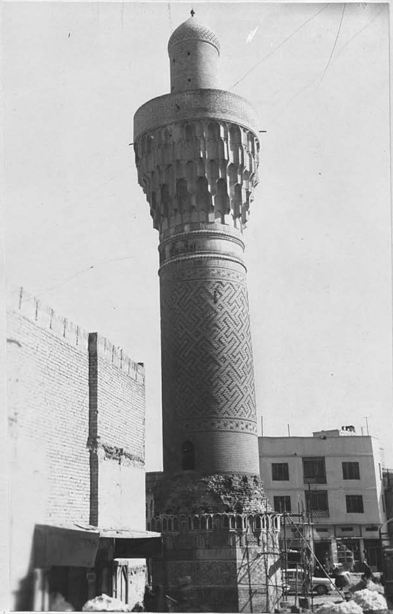
62. Baghdad. The minaret of Sūq al-Ghazl: brickwork of the shaft and the upper part after restoration.
