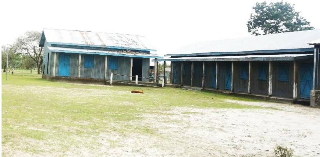
Picture 10: Newly constructed primary school in Bashaini Char (notice the closed doors and windows)
