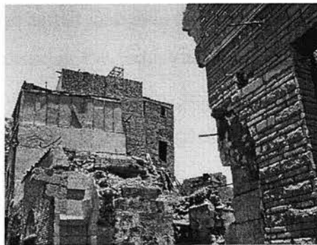
Ill. 6.25: Insensitive demolition of Wikalat al-Zaitun has a negative physical impact on the surrounding residential buildings in al-Tumbakshiyya Street.
