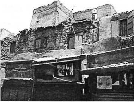
III.2.8: A collapsed Rab' (collective housing units), al-Tabbana Street, al-Darb al-Ahmar the building was altered having hovels to house those who lost their units, and it is typical situation to have only the shops that still function.
