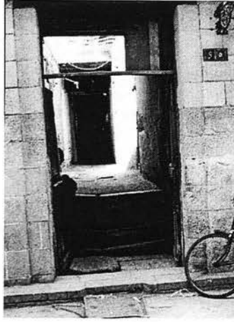
Ill. 6.22a: Painting the houses in al-Darb al-Asfar Street was the main goal regardless restoring them or dealing with their threatening, dilapidated condition.
