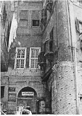
III.2.7: A nineteenth century apartment building, see the unsuitable finishing material adorning the ground floor and the modern building in front permitting limited illumination.
