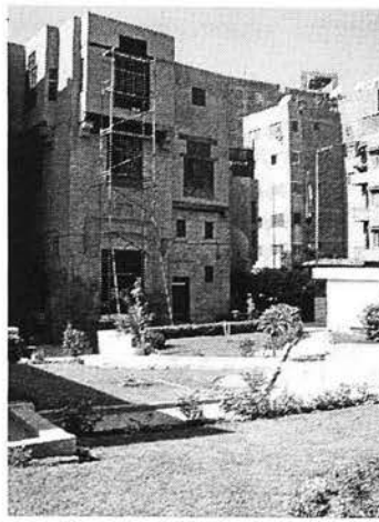
Ill. 6.13: The open area behind al-Kirtliyya House, historical mansion under restoration, in Ibn Tulun Area.
