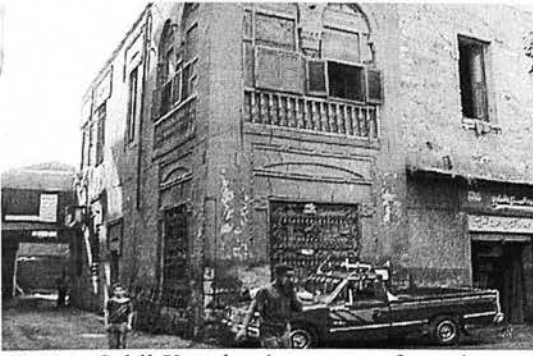
III.2.1: Sabil-Kuttab (a water fountain surmounted by an elimatory school built ca. seventeenth century) the inhabitants of the neighbouring building added the upper part illegally to their apartment.
