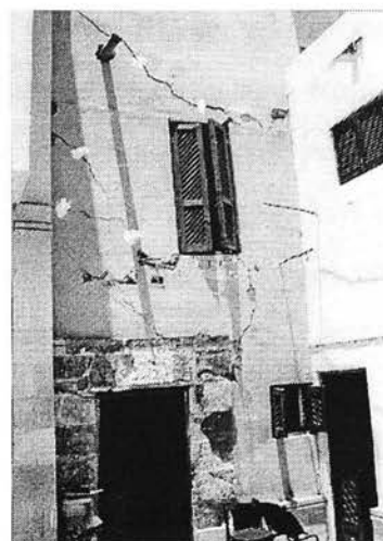
Ill. 6.9b: Lethal cracks left on the wall-baring houses in Qasr al-Sham Area as a result of insensitive construction work.
