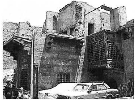
III.2.4: A registered monument (traditional mansion) in a very ruinous condition, Al-Tabbana Street, al-Darb al-Ahmar
