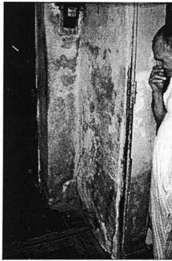
Ill. 6.22b: Wall-baring houses with lethal cracks that can collapse are only painted; this example is located at 4 Atfat al-Darb al-Asfar, off al-Darb al-Asfar Street, where the historical houses are located.
