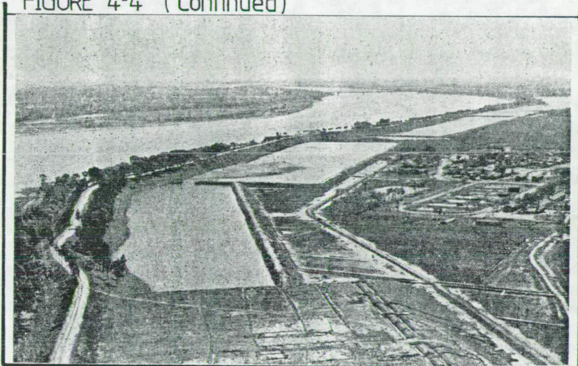
(c) Settling ponds for dyke consolidation by warping. Source: RHWCC, Eds., 1979, p. 255.
